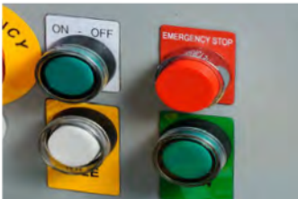
Control panel labels
