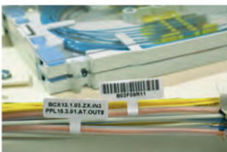
Fibre optic cable markers
